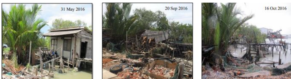
Figure 3. Impact of coastal erosion to the residential property at Bagan Pasir, Selangor (Adapted from [13])
