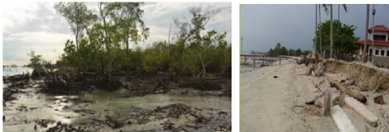
Figure 4. Coastal erosion and its impact to the coastal infrastructures at Batu Pahat, Johor (Adapted from [14])
